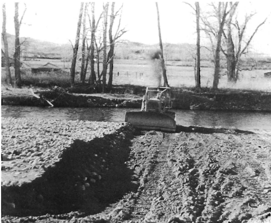
Figure 2.—Desecration of a stream bed associated with road construction.
