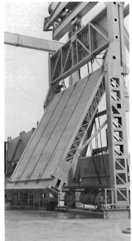
Figure 17.—Traveling screen shown in operating position on the deck of Little Goose Dam. Hydraulically operated arm is withdrawn to permit lowering of screen through gatewell slot.
