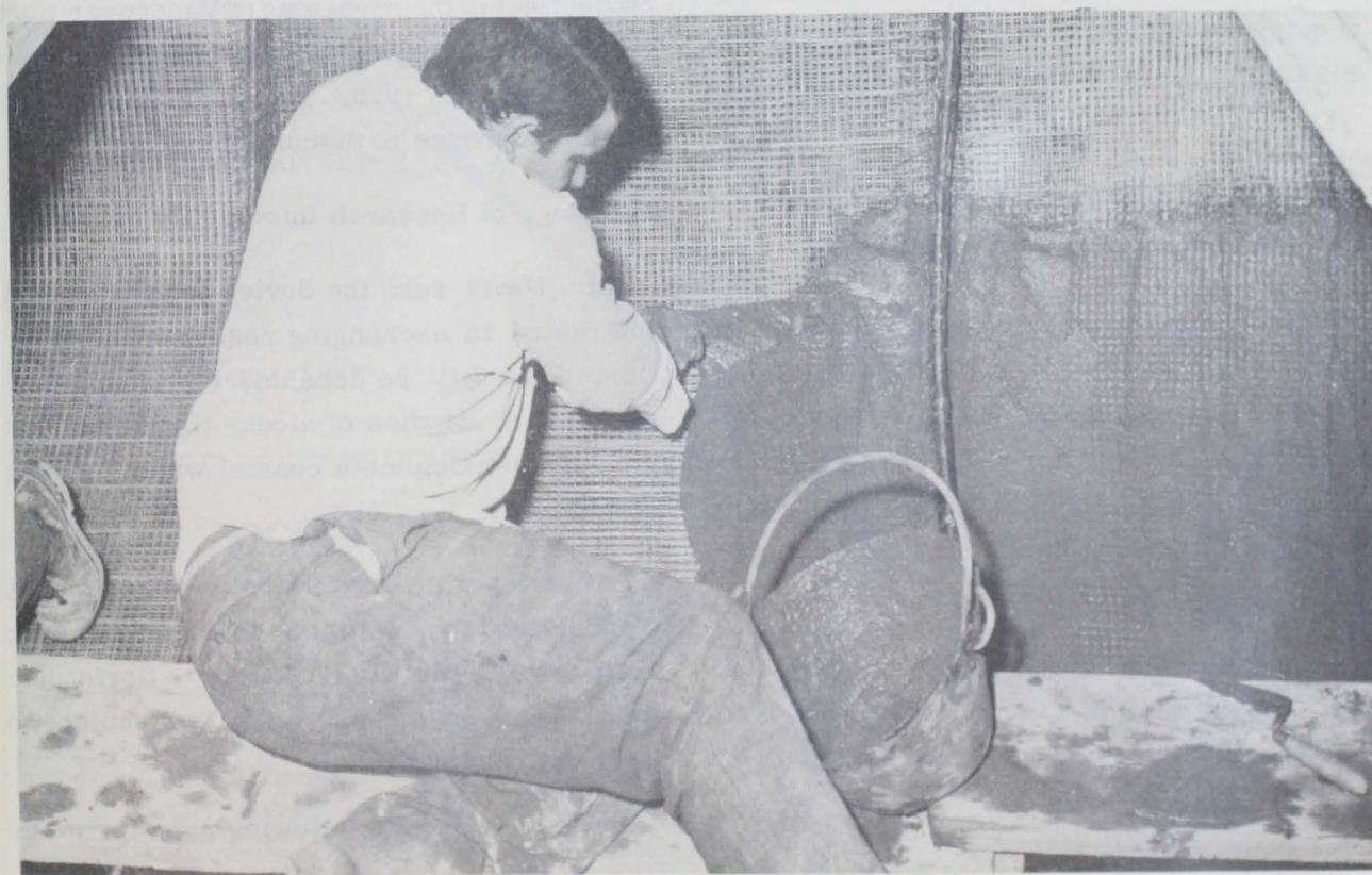
Fig. 2 - Plastering a ferro-cement boat hull. To assure good penetration, the mortar is applied from inside, forced through reinforcement, and smoothed on outside. (FAO photos)
