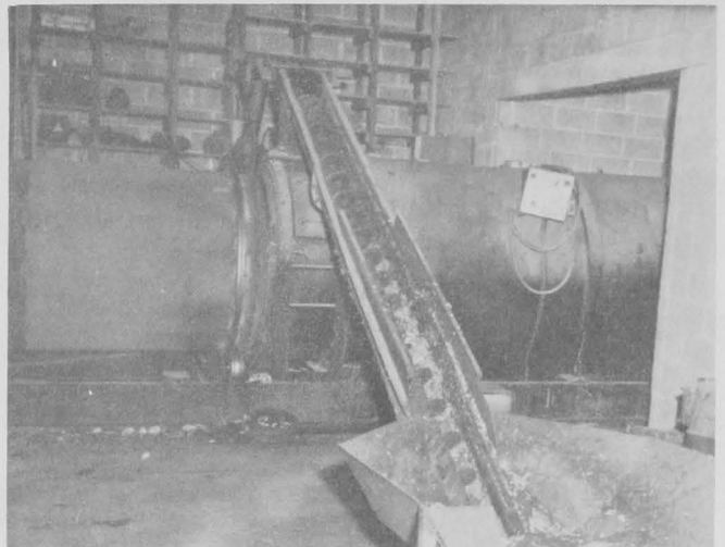
Fig. 16 - Many of the larger plants solve the problem of waste disposal by converting the waste into a salable product by use of a crab-scrap dryer. Waste from the debacking operation and the picking tables is dumped into the big hopper (foreground) and carried into the rotary dryer by means of a screw conveyor.
