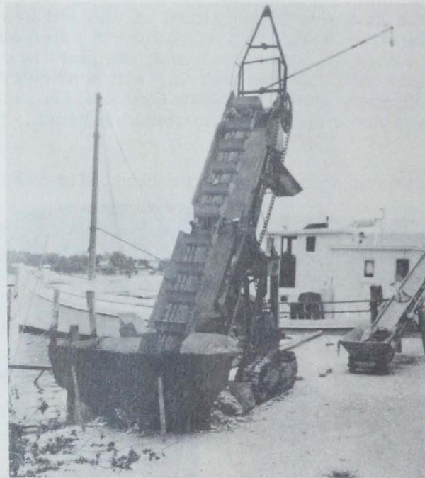
Fig. 5 - The bucket-loading conveyor is on a halftrack, is self-propelled, and includes a small lifting boom located on top. The commoner type of portable loader, seen in the right background, is mounted on large wheels and is moved by manpower.
