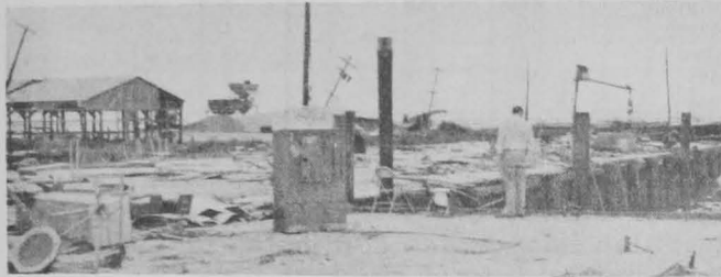
Fig. 2 - After Hurricane "Carla," this is what remained of a crab-picking plant located on this bulkhead in Palacios, Tex.
