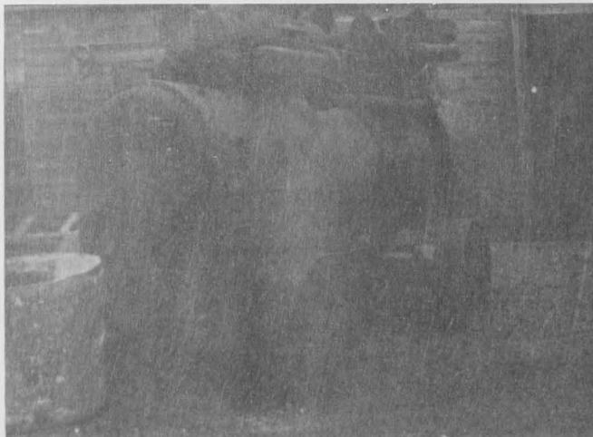
Fig. 30 - Portable coal-fired steam boiler used at October Combine fish-meal plant.
