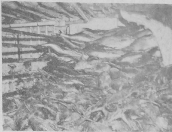
Fig. 5 - Starboard, or right side, of Jo Ann's hold. At the top are the small pipes (crisscross above the larger coils) which spray water on the larger coils (notice that they still have ice on them).
