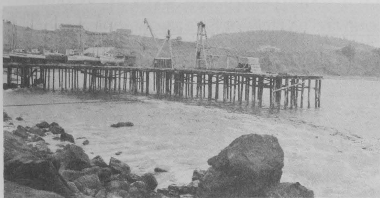
FIG. 3 - END OF DOCK, SHOWING THE DERRICK AND A PILE DRIVER. (THE CABLE IS THE SAME ONE THAT IS SHOWN IN FIG. 1.)
