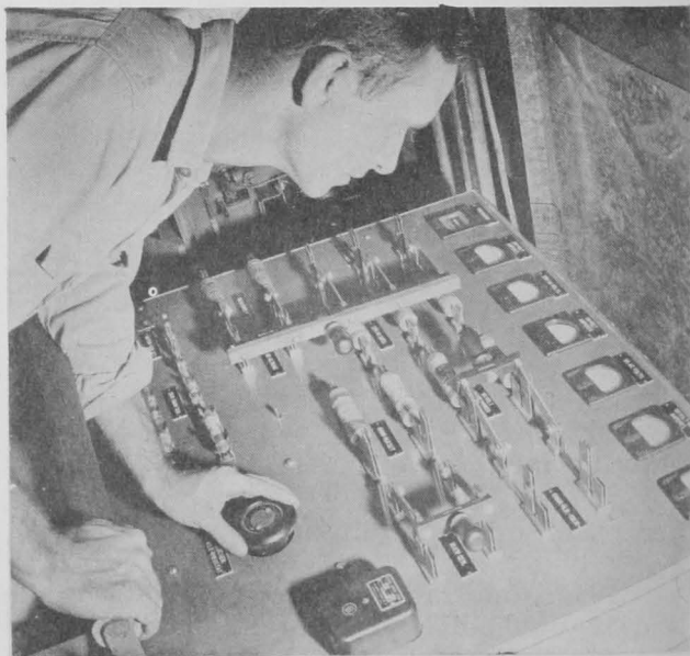
Fig. 9 - View of power-distribution panel, showing 110 v. a.c., 110-v. d.c., 32 v. d.c. controls, and isolation transformer.
