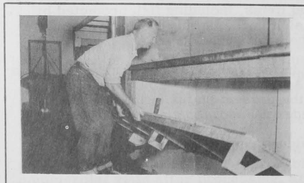
Fig. 2 - Placing grate in working position. Note the wooden stop on the left-hand wall.
