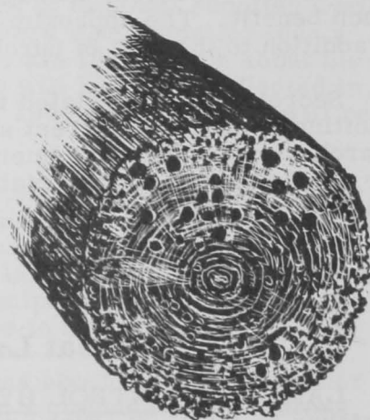
Large tubes made by Bankia and small tubes made by Teredo on piling.
