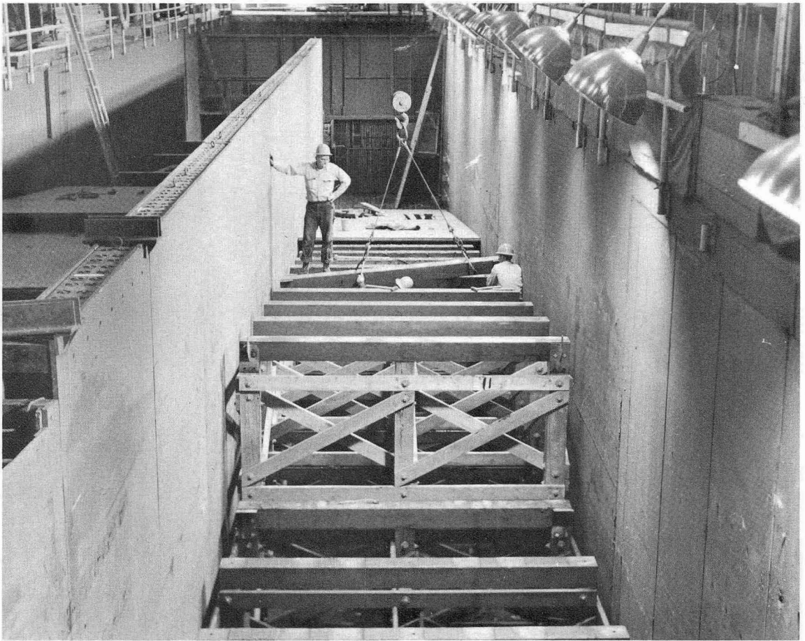
FIGURE 3—Installation of floor frames for the 1:8-slope fishway. A section of floor is in place at the lower end of the fishway.
