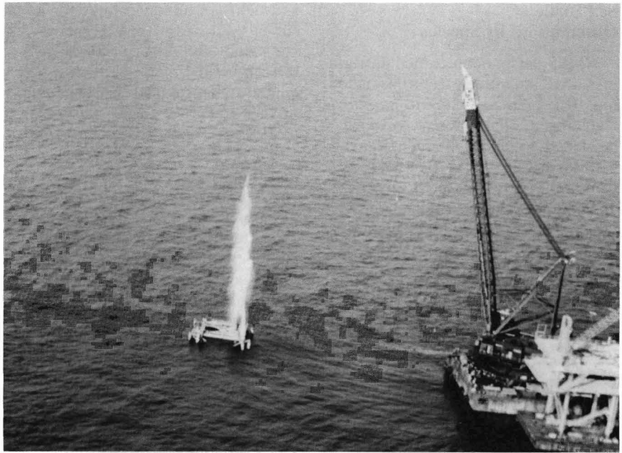
A geyser of water blasts from a piling during the explosive removal of an offshore platform. Plastic explosives are detonated inside the hollow legs of the platform at a depth of 5 m below the sea floor. The part of the platform standing above water, referred to as the deck, has already been cut with torches and lifted onto a barge (lower right) by a large crane.
