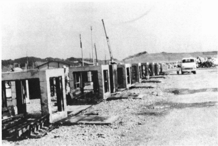
Figure 1.—Japanese concrete cube reef units (sides = 2 m) being built in Chiba Prefecture, Japan.
