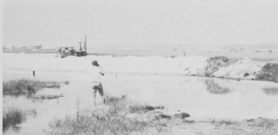
Close-up view of dredge and fill operation in progress for housing and industrial development.
