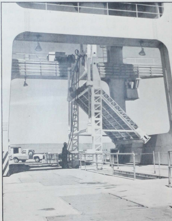
Figure 3.—Inclined traveling screen shown in operating position on deck of dam. Hydraulically operated arm is withdrawn to permit lowering of screen through gatewell slot.
