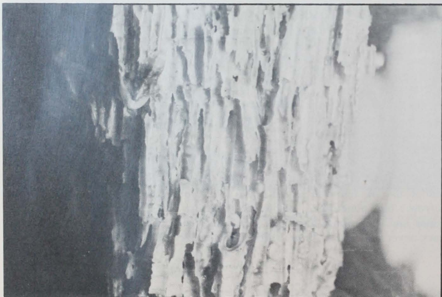
(Left.) Section of wooden structure riddled by shipworms. Photograph by Dr. D. B. Quayle, Fisheries Research Board of Canada.
