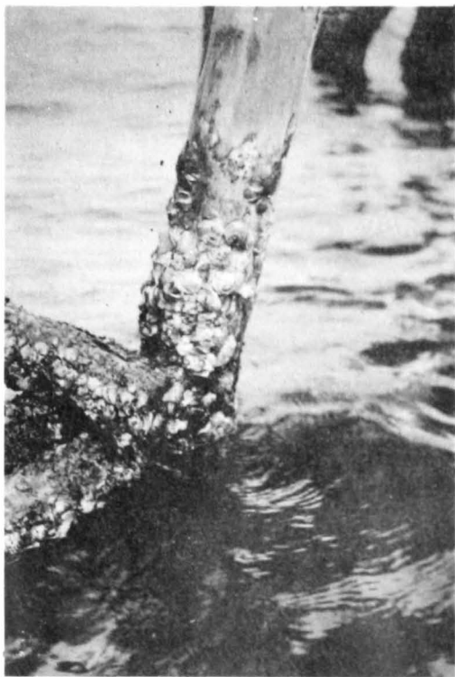
FIG. 10 - THE PROLIFIC SETTING OF THE MANGROVE-TYPE OYSTER ON THE PILINGS OF THE FISHERY WHARF IN THE MONROVIA FREE PORT IN DECEMBER.
