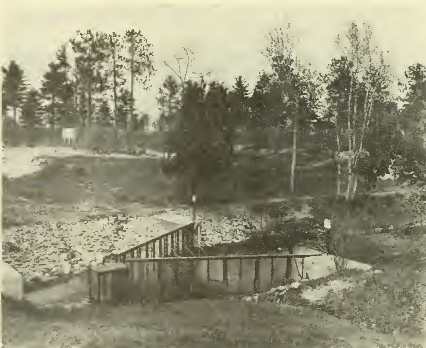
Figure 5.--Portable-type weir and trap in Carp Creek, Presque Isle County, Mich., after installation of permanent sills, trap base, and abutments of concrete.
