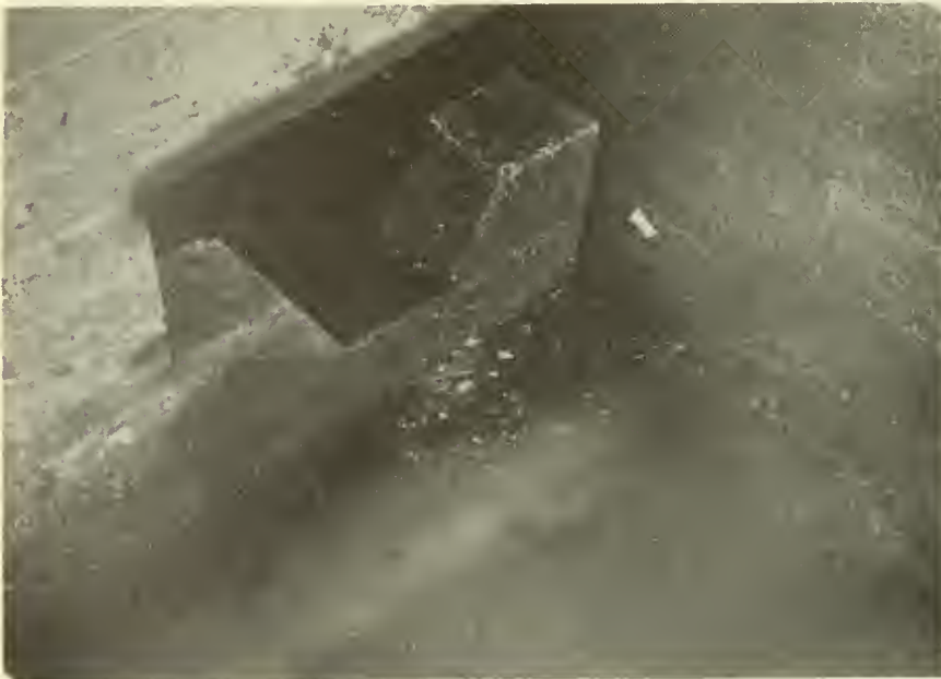
Figure 11. -- Notched Weir. Note the unusual thickness of the weir and the sloping floor of the notch. The downstream edges of the notch have a 2-inch bevel.
