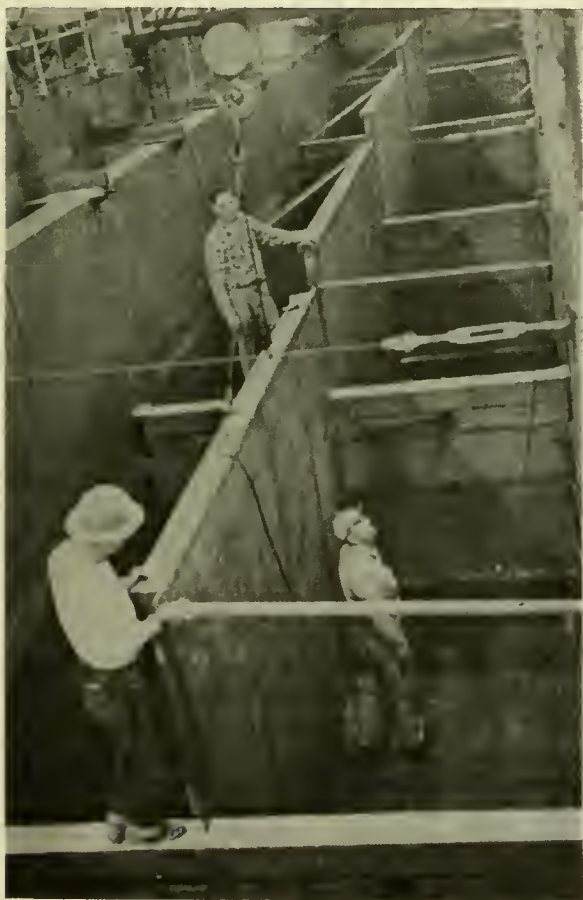
FIGURE 1.--INSTALLING PARTITION WALL TO CREATE A 6-FOOT WIDE FISHWAY FOR THE CAPACITY TESTS.
