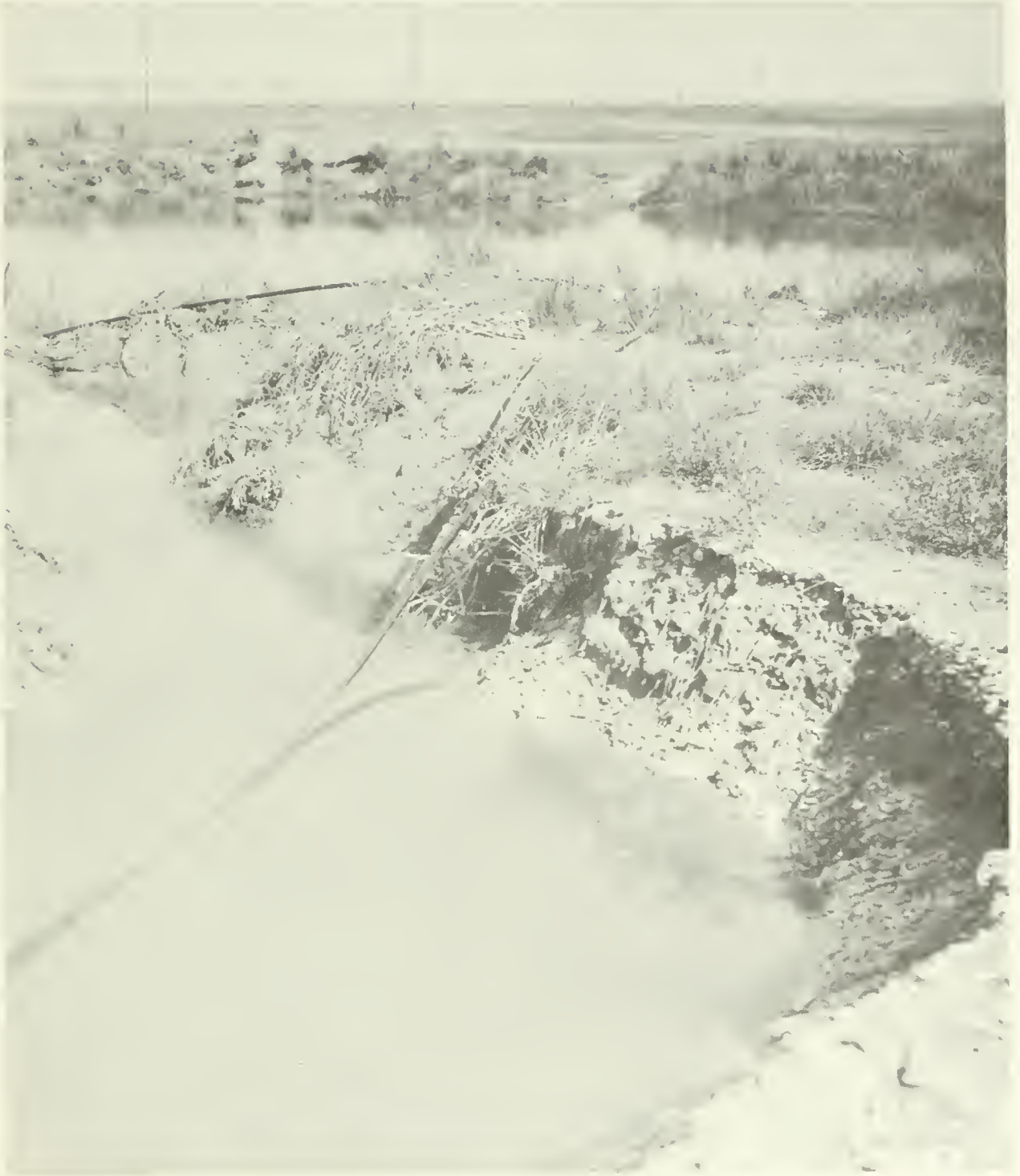
Figure 5.--Flooding of a rearing pond by an excessively high tide destroyed a bank unprotected by transplanted marsh-grass.
