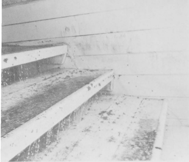
Figure 9. Interior of the splash tower for deaerating sea water.
