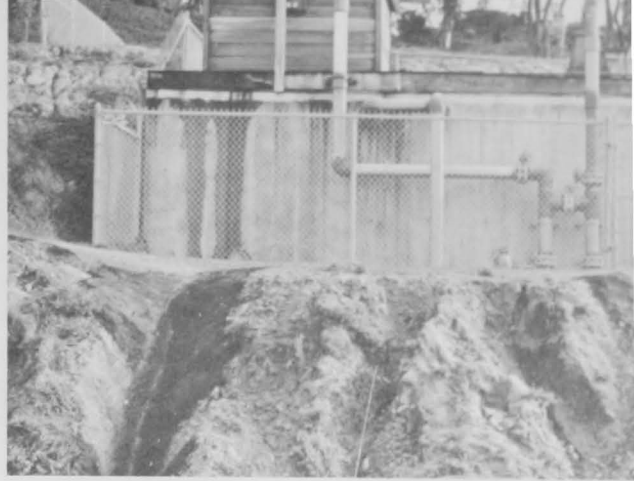
Figure 8. Storage tanks on a hill directly above the experimental aquarium. Two pipes enter the tanks from above, but only the one to the large deaerating tower is used at present after water arrives by either of the two pipes emerging from the ground on the right.
