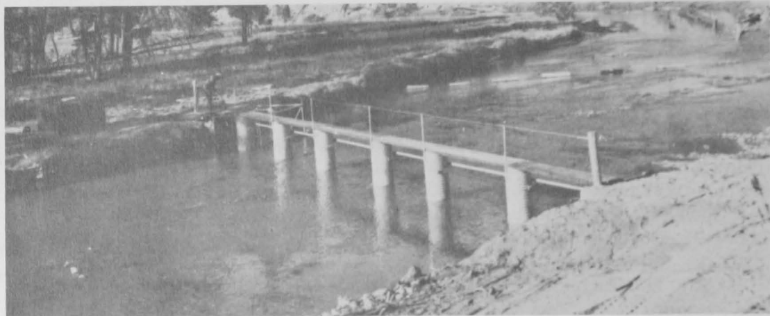
New fish traps were constructed by the National Park Service on three tributaries of Yellowstone Lake to serve as counting weirs. Photo: Ron Cotten.
