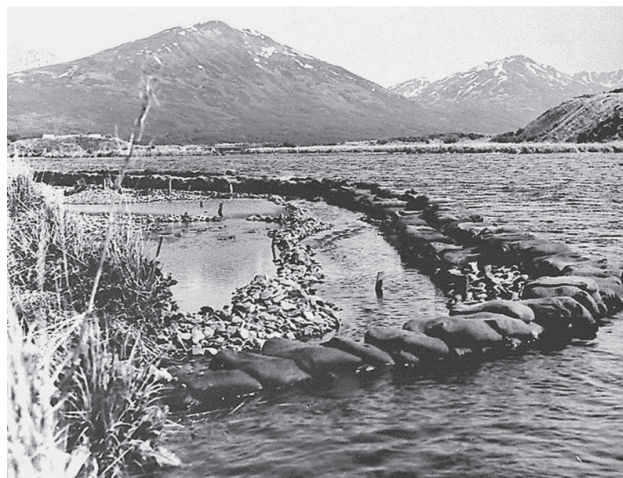
Coffer dam for construction of a two-way permanent salmon counting weir, upper Karluk River, June 1949. (Richard F. Shuman, Auke Bay Laboratory, Auke Bay, AK)
