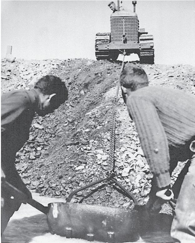
Using a slip scraper and Cletrac tractor to excavate the footing for a two-way weir, upper Karluk River, June 1949. (Richard F. Shuman, Auke Bay Laboratory, Auke Bay, AK)
