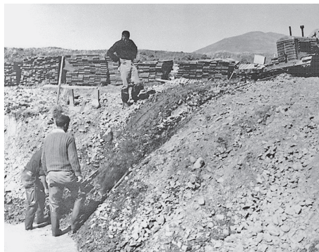
Excavating footing for a two-way weir, upper Karluk River, June 1949. (Richard F. Shuman, Auke Bay Laboratory, Auke Bay, AK)
