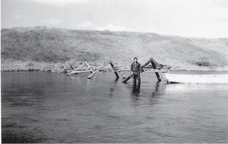
Installing the Karluk River weir, Portage, 1942. (Allan C. DeLacy, from Catherine J. DeLacy, Seattle, WA)
