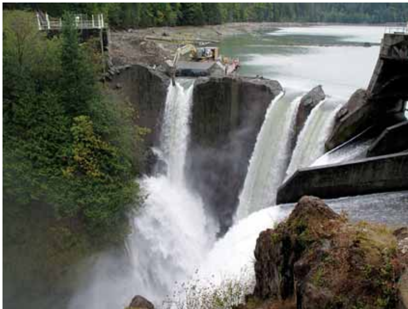
The Glines Canyon Dam, in Washington State, in the early stages of being dismantled.
